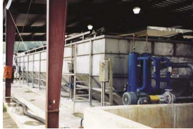
This VanAire DAF is installed at a chicken slaughter plant with a chemical treatment program. DAF effluent is typically under 100 ppm BOD, 10 ppm FOG/ TSS.
